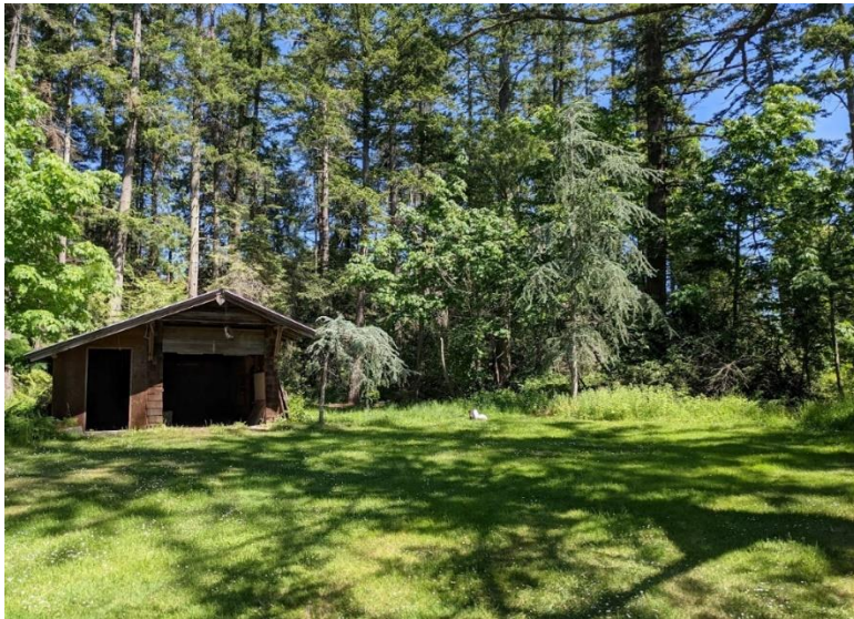
Figure 4: Dilapidated shed in the grassy area of Denham Till - remnants of an agricultural history
